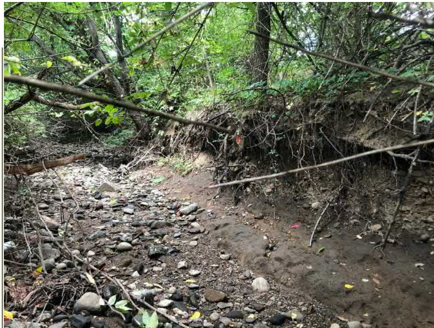
Looking Upstream. Toe and Bank Erosion
