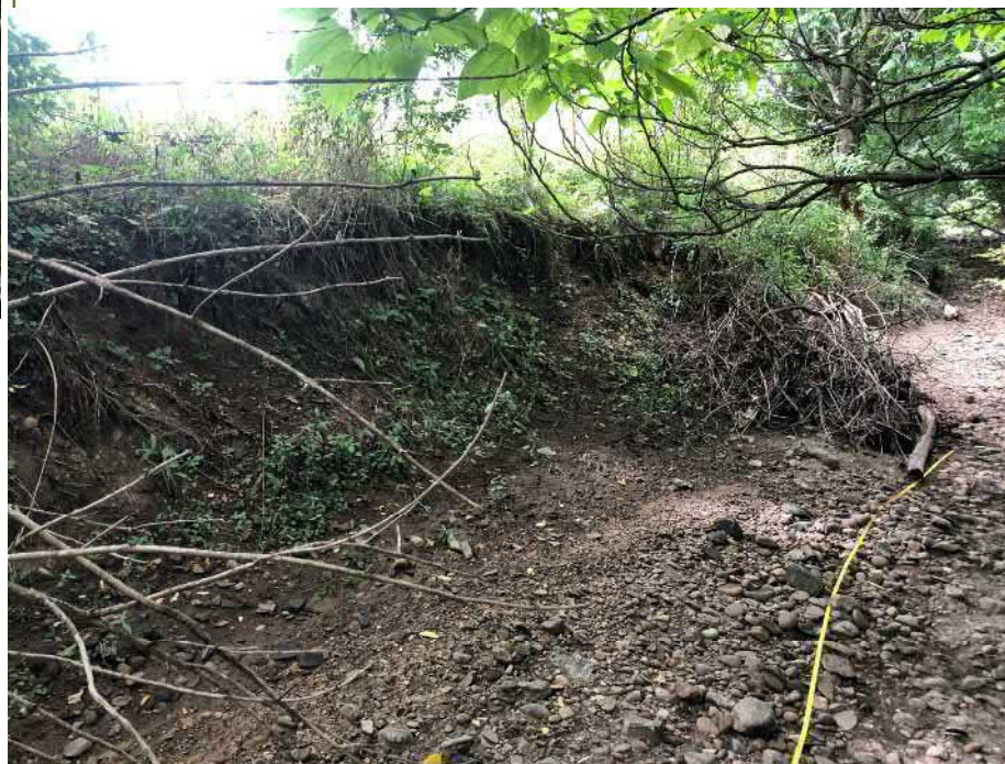
Looking Upstream. Toe and Bank Erosion
